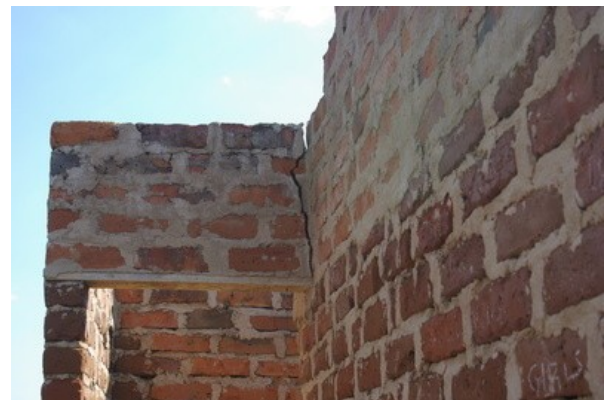
Figure 2: Crack at girls' entry
