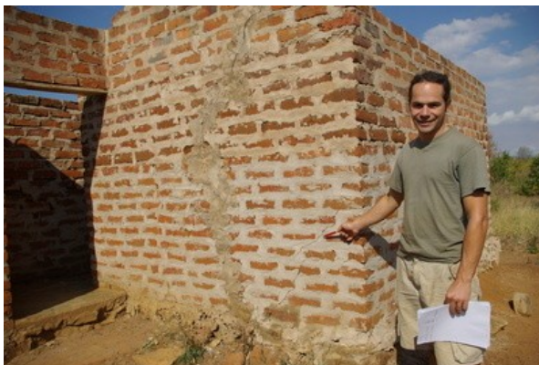
Figure 1: Cracks in girls' toilet building
